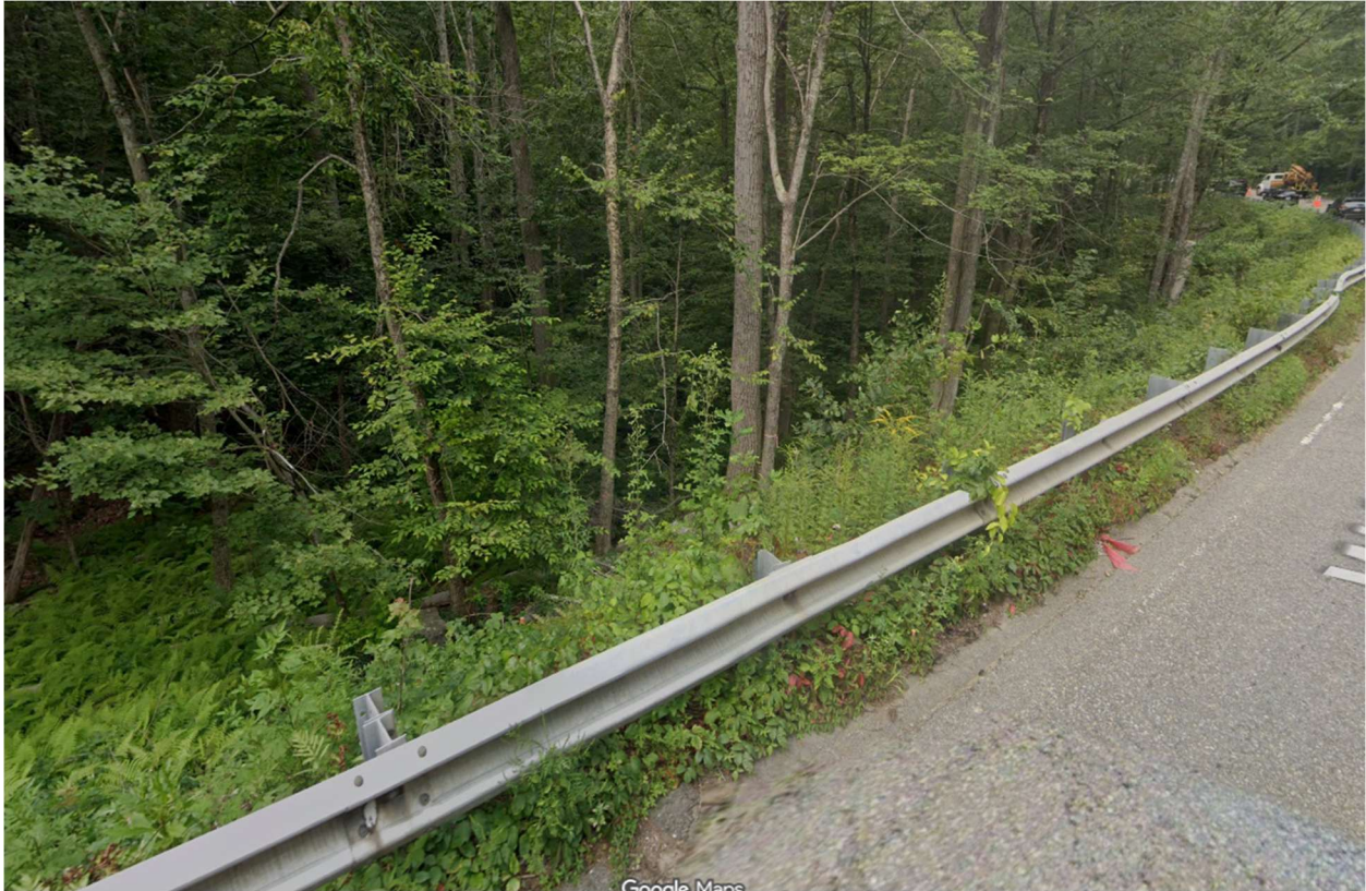
Example of significant grade behind the guardrail.
