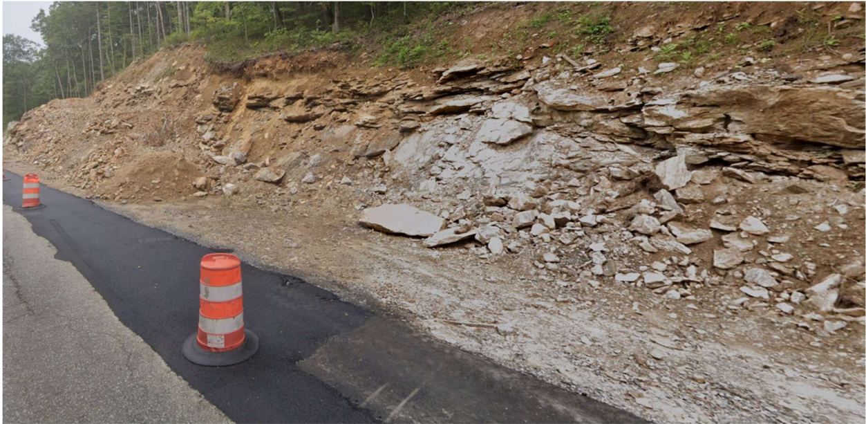
Significant rock ledge and grade issues.
