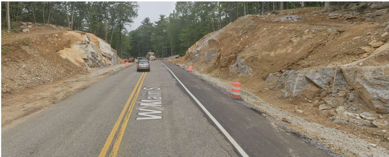
Significant rock ledge on both sides of the roadway.
